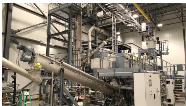
BIOGREEN pyrolysis plant
